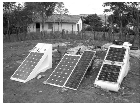
Figure 10: From left to right: Enhanced I-SHS (smaller version than Fig. 9) equipped with a 32 cell module, a reference module of the same type, a conventional 36 cell module, and an I-SHS of 2002 as shown in Figs. 5, 6 (Serra de Baturité, Ceará, 2005).
