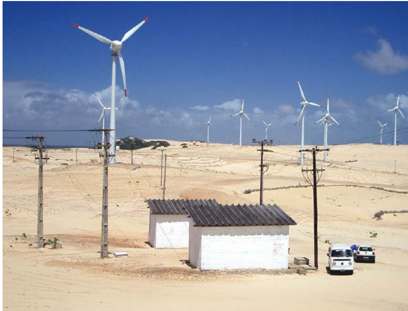
Figure 6: Grid connection points (2 x 5 MW, in the huts) to the public grid of COELCE (to the left) at the Prainha wind park (from the right).
