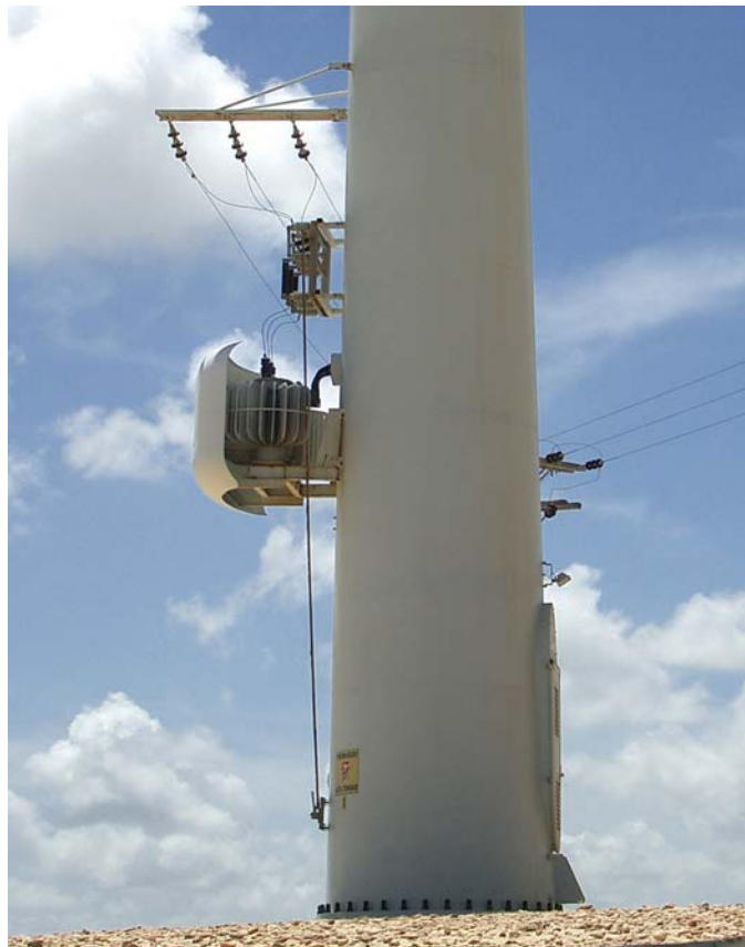
Figure 5: A 500 kW transformer (380 V to 13.8 kV) attached to a single E 40 wind power converter.
