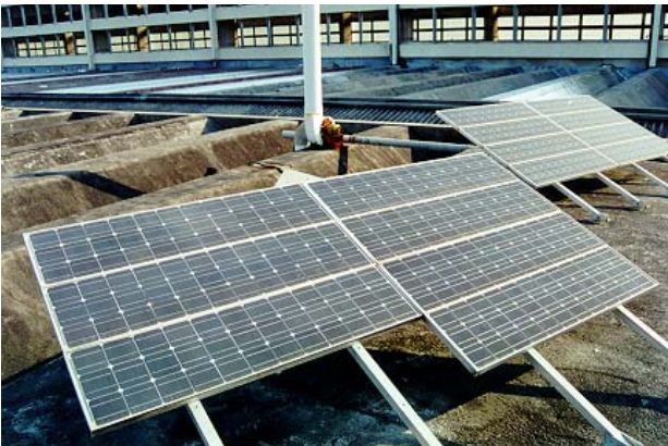
Fig. 3. 800 W p PV-generator at Laboratorio Fotovoltaico, UFRJ-COPPE.
