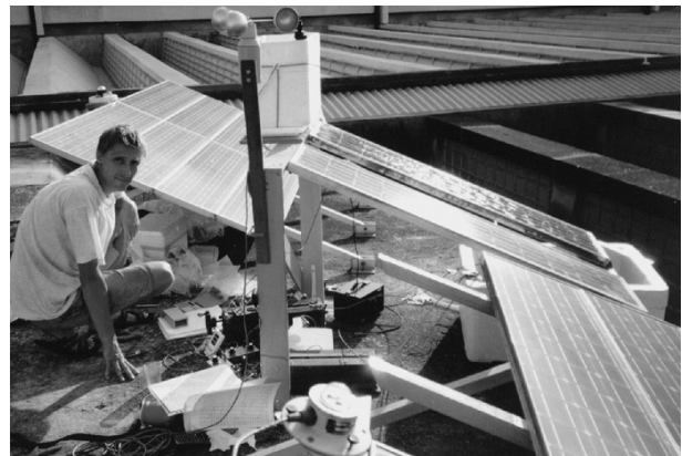
Fig.4. Example of recent research at PV-Labs UFRJ-COPPE: Increasing the yield of a PV-generator: Lower operating cell temperature and less reflection losses by a frontside water film .
