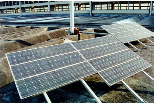
Fig. 3. 800 W p PV-generator at Laboratorio Fotovoltaico, UFRJ-COPPE.
