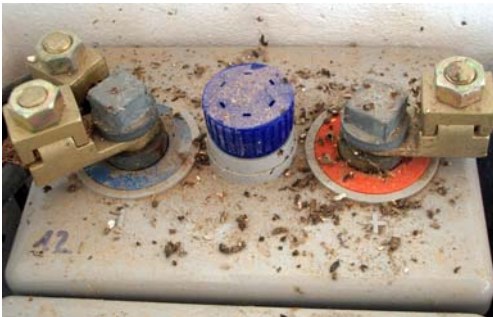
Figure 5: New battery after a couple weeks: rats liked the place, leaving excrements.
