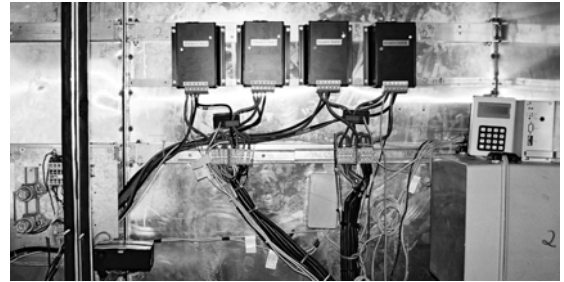
Figure 5: Charge controllers with the Hall-effect current sensors (center), enabling a current-balance for the batteries, and at the satellite transmission device (on the right) during installation.
