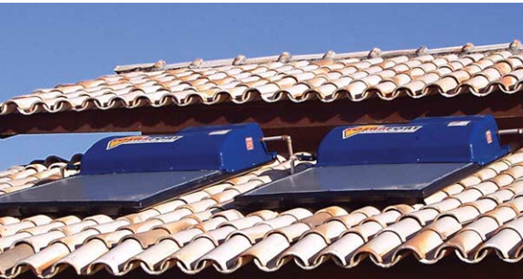
Figure 2: Brazilian solar thermal systems; collectors with integrated storage, substituting electrical showerheads.
